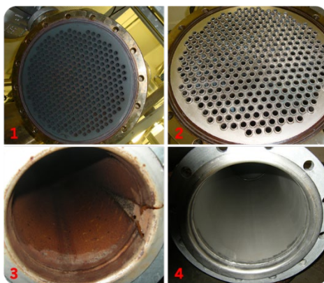
Fig. 2. Tube plate of a steam raising unit before (1) and after (2) derouging. Pipe system before (3) and after (4) rust removal with new pH neutral formulations with NTZ clean neutral .
